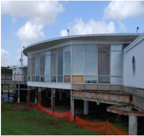
2008 Exterior after Hurricane Ike (photo courtesy of SWCA)
