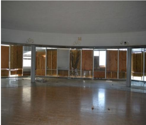
2008 Interior after Hurricane Ike (photo courtesy of SWCA)
